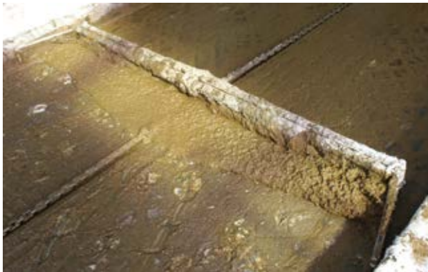
Ensure the scraper runs frequently enough to keep the volume of scraped slurry from overflowing onto the beds.
